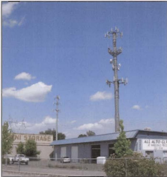
Hartnell Avenue cell towers
